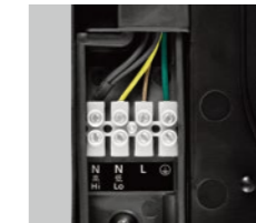
Power Supply Terminal
