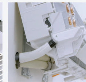
More open working spaces provide easy view and unobstructed access to setup drain hose and piping.
