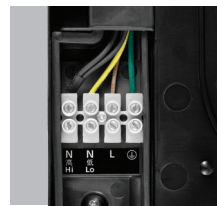
Power Supply Terminal
