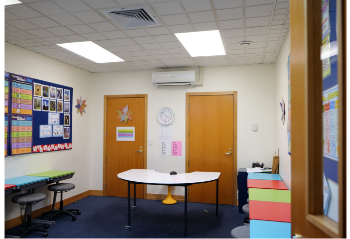
air-e ceiling mounted nanoe™ X generator installed in St Cuthbert's College's classroom.
