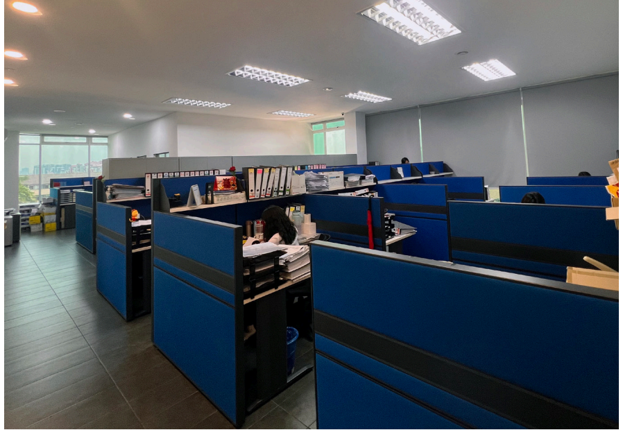
air-e nanoe™ X generator installed in a work space to provide purified air.
