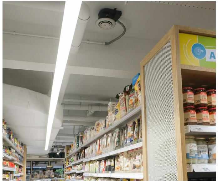
Neat installation of ceiling-mounted air-e nanoe™ X generator.
