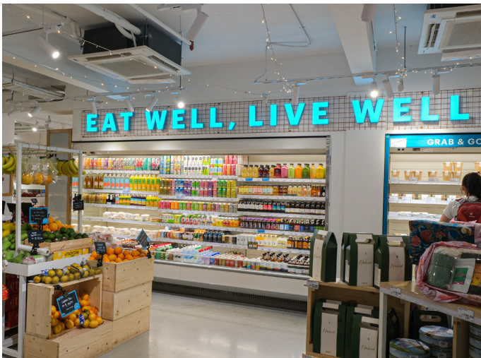
Cassette air conditioner installed in Qra The Five.
