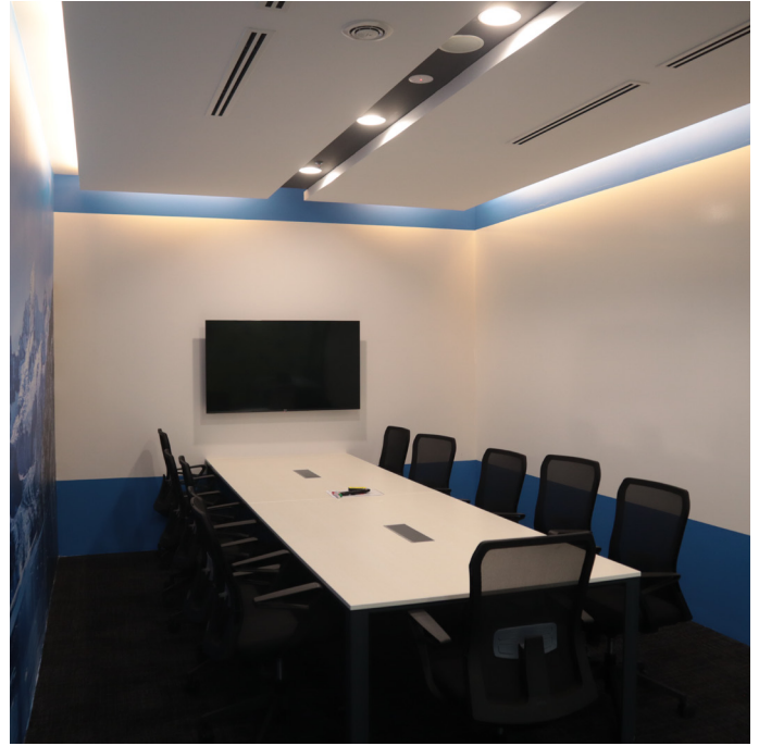
air-e nanoe™ X generator installed in a meeting space.
