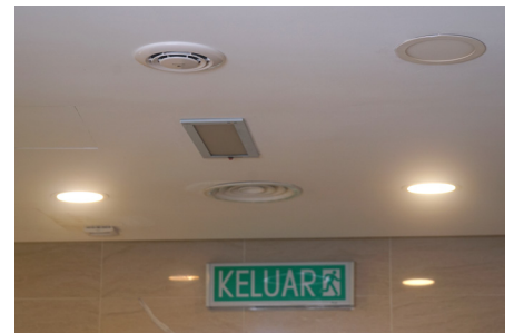
Neat installation of air-e nano e ™ X generator.
