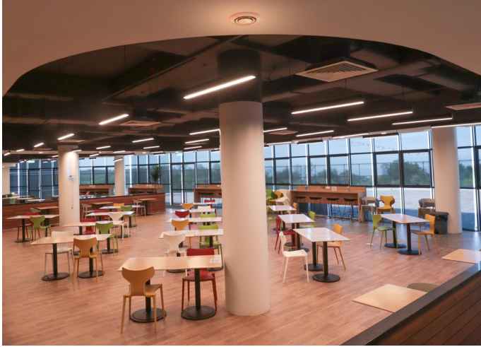
air-e nanoe™ X generator installed in a campus' cafeteria.
