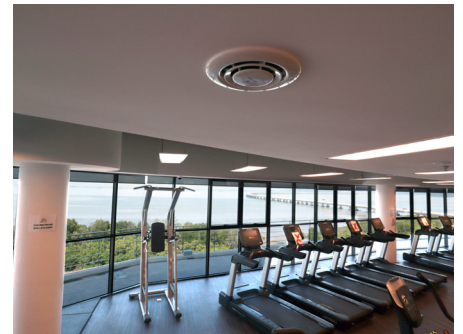
air-e nanoe™ X generator installed in a campus' gym facility.
