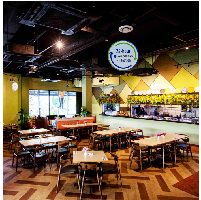
air-e nanoe™ X generator installed in one of the outlets in D' Network F&B.
