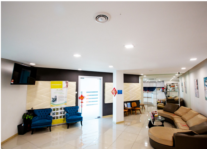
air-e nanoe™ X generator installed in a clinic waiting area.
