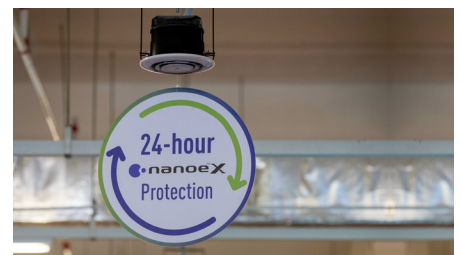
air-e nanoe™ X generator installed in D'Network is powered by solar and is in full operation for 24 hours.
