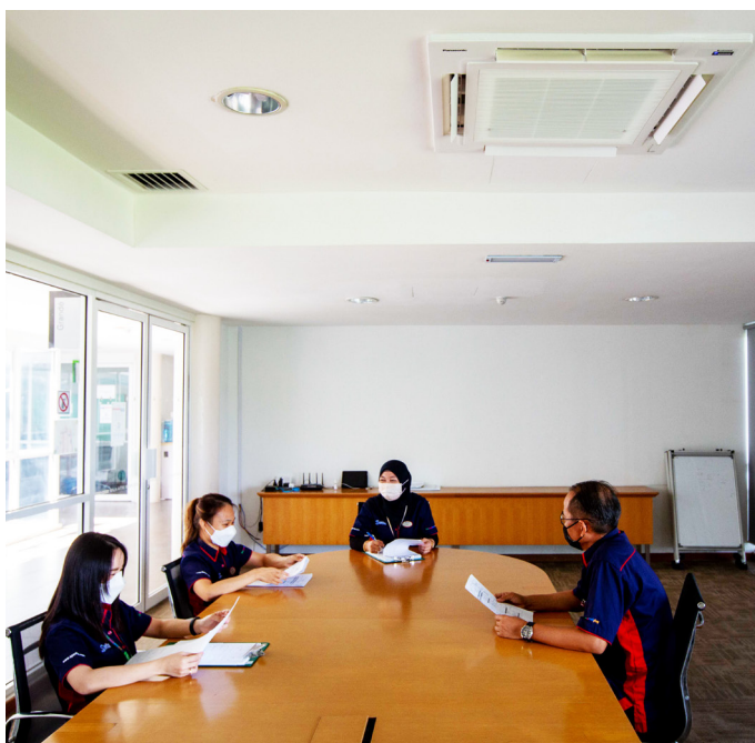
Cassette air conditioner equipped with nanoe™ X installed in Setia Alam Welcome Centre's meeting room.
