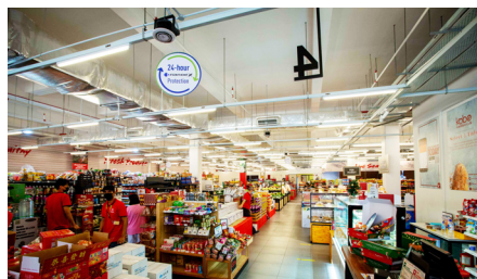
air-e nanoe™ X generator installed in the grocer store.
