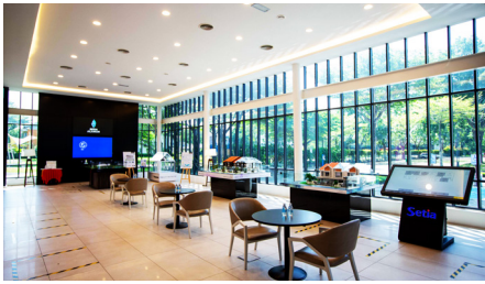
air-e nanoe™ X generator installed in Setia Alam Welcome Centre.
